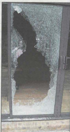
EXPENSIVE – Some of the damage caused at All Saints Church
